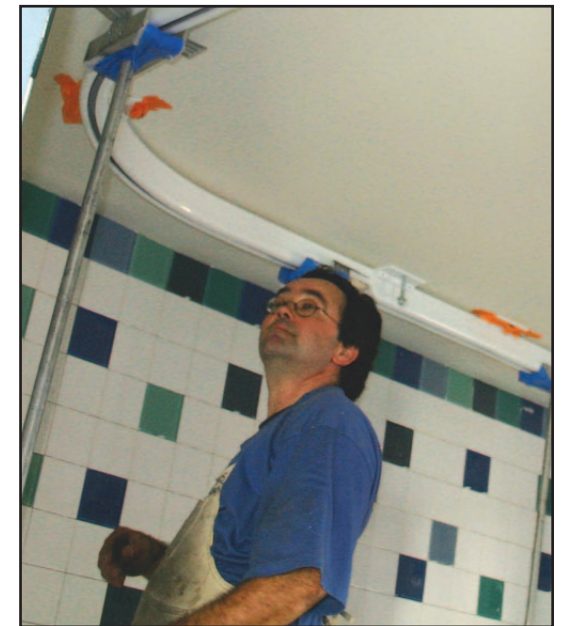
Craig Coogan of Lift & Transfer Specialists lends a helping hand, installing the SureHands lift system on the popular TV show Extreme Makeover: Home Edition .
